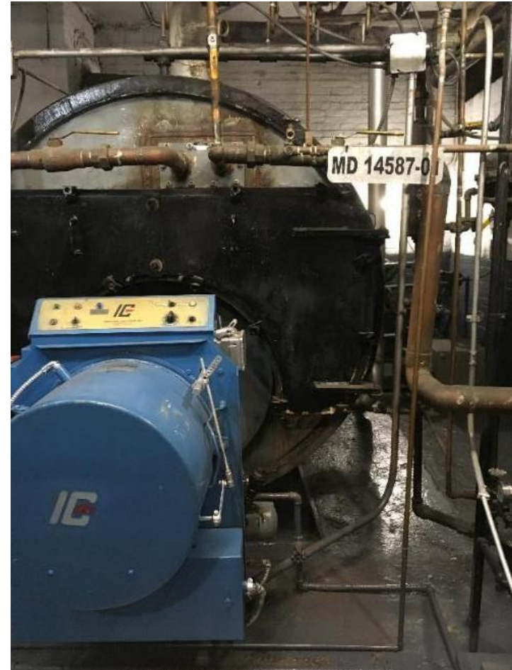
Old, inefficient boiler
